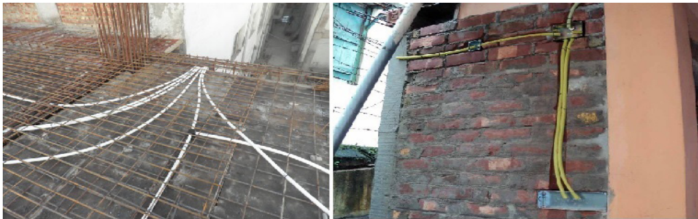
Fig. 4.1.15: Concealed Conduits in Brick Wall
